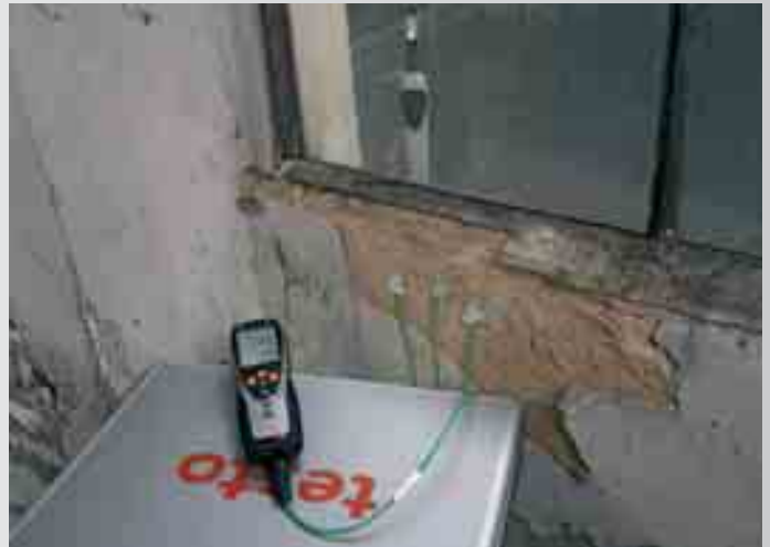
Measures the U-value in a wall in need of renovation using U-value and wireless temperature/humidity probe (alternatively conventional temperature probe also)
