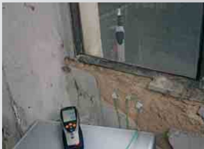
Measuring the U-value at a wall in need of repair with a U-value and wireless temperature/humidity probe (also possible with a temperature probe)
