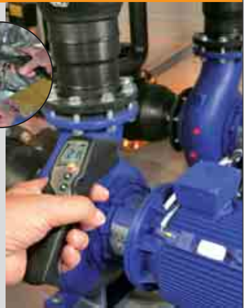
Checking temperature on a compressor
