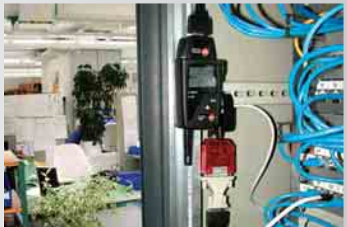
Read out the data stored in the logger via the PC network using the Ethernet adapter
