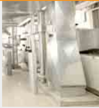
Monitoring ambient conditions in ducts
