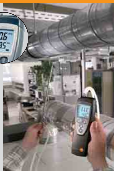
Measuring process air
