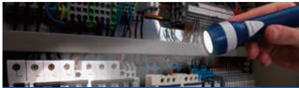
Erroneous circuit-breaker activation
